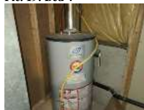
Pic. 23: Hot water tank
