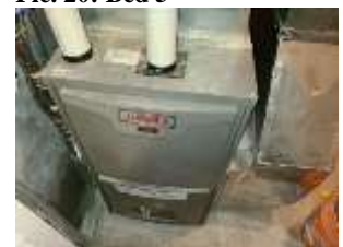
Pic. 24: Gas furnace 2018
