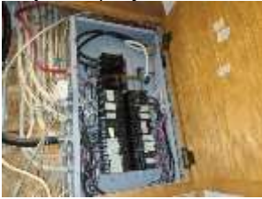
Pic. 25: 100 amp breaker panel – front cover missing
