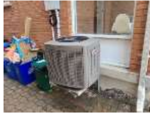
Pic. 2: AC unit 2019
